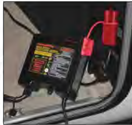
70 amps is plenty of juice for powering systems in small jets. The VDC BatteryMinder, top, is integrated with the GPU but can be purchased separately and hardwired for easy plug-in.
