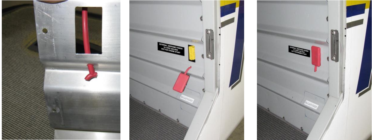
Opening in baggage closeout panel. Finished installation showing connector exposed and covered. Beautifully done.
